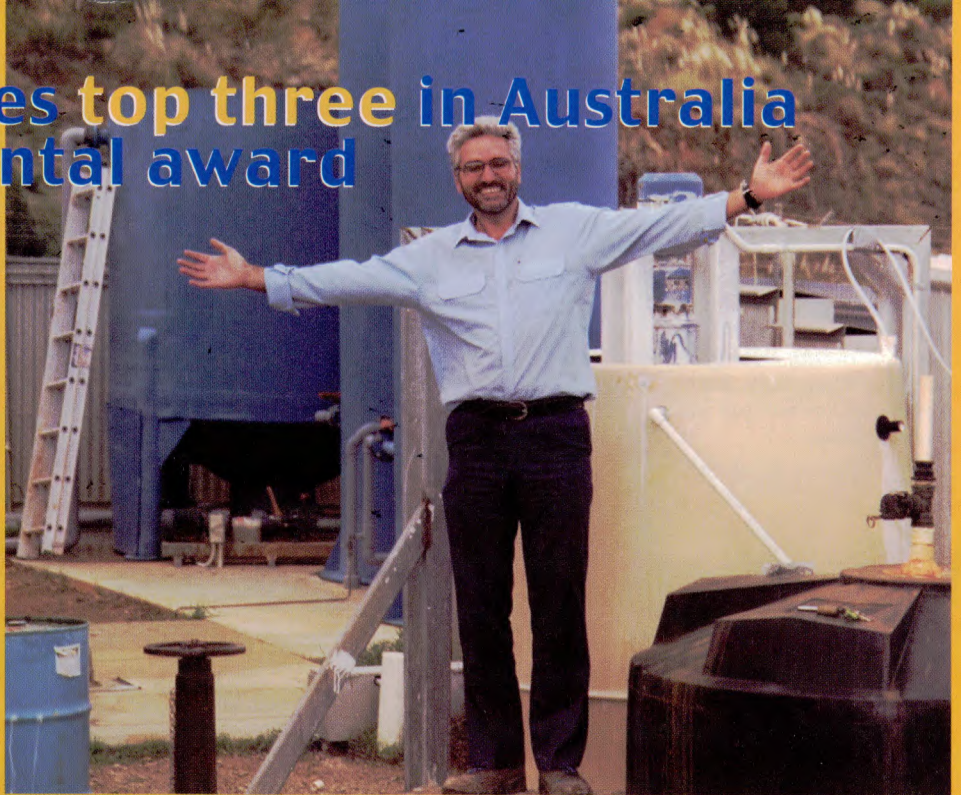
City of Cockburn Landfill Supervisor - Andrew Stevenson shows off the new leachate treatment plant.
